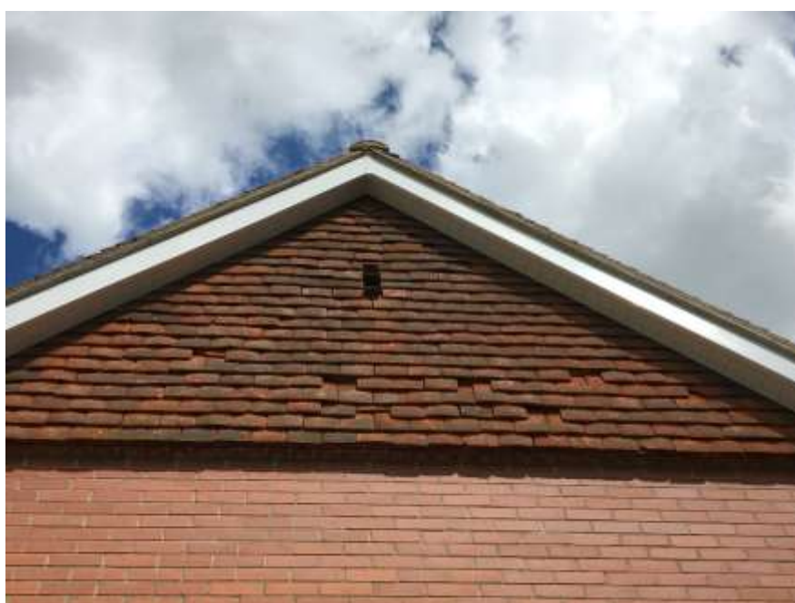
Photograph 4: Missing hanging tiles and gaps under hanging tiles that offer suitable roosting habitat for bats
